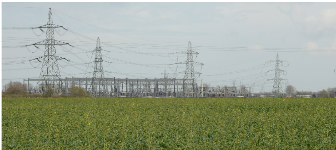
Img 3 - Creyke Beck Substation, approximately 180m east of the OnSS site (Source: Orsted)
